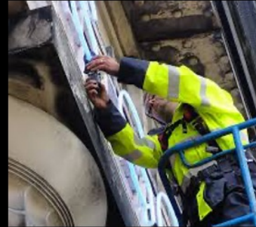
Technician from Neon Circus fabrication studio repairs failed units Photo: Neon Circus
